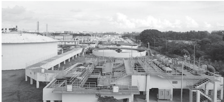
Fig 2: KCVP Treatment Unit
